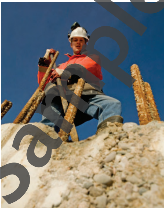
A rock falls from the edge of this excavation, but lands on the ground without causing injury or damage - a near miss
