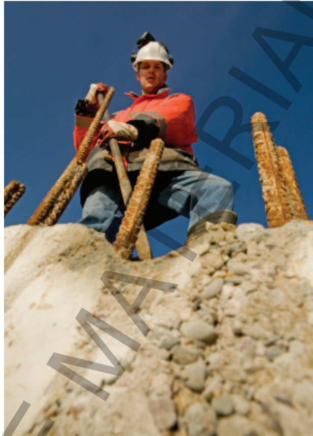
A rock falls from the edge of this excavation, but lands on the ground without causing injury or damage - a near-miss
