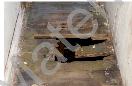
A collapsed floor could lead to a worker being injured
