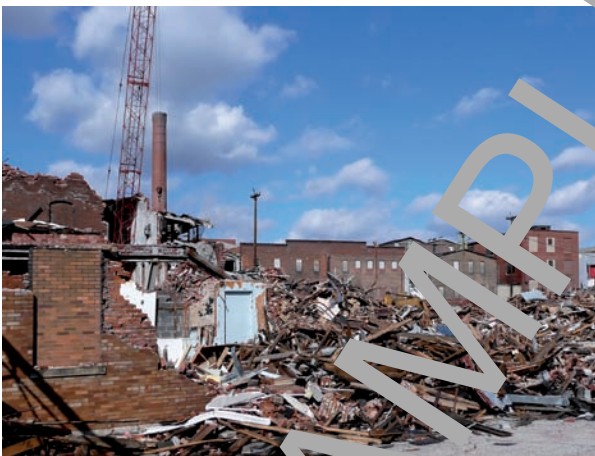
The possible result of unsuccessful explosion prevention techniques
