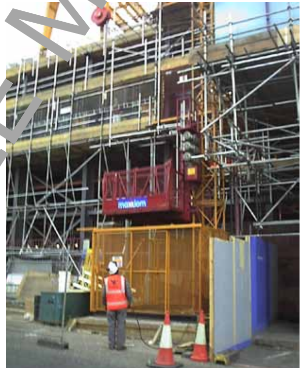
Electric hoist moving load
