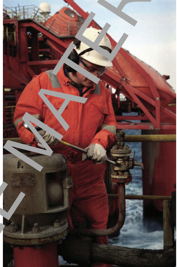
Engineer carrying out condition-based maintenance
