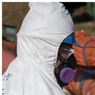
A worker wears a half-mask respirator to seal asbestos lagging around a pipe
