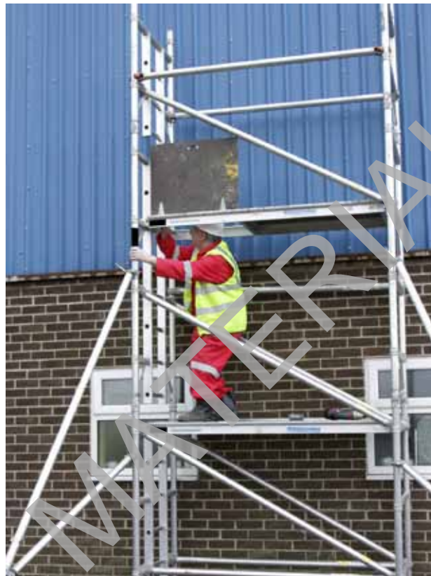
A worker gains entry to the top of a tower scaffold using internally fixed ladders, through internal trapdoors. This tower has outriggers attached.
