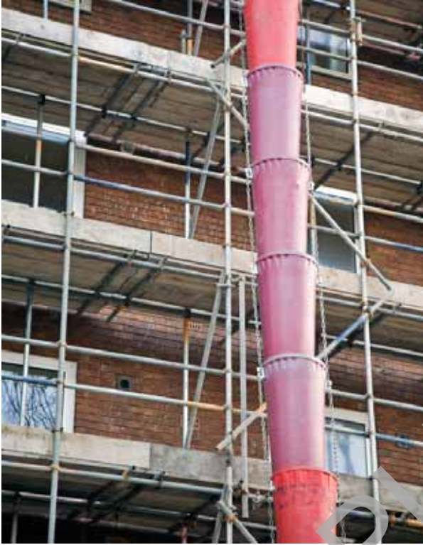
An independent tied scaffold with guardrails and toeboards, and a debris chute for safe removal of rubble
